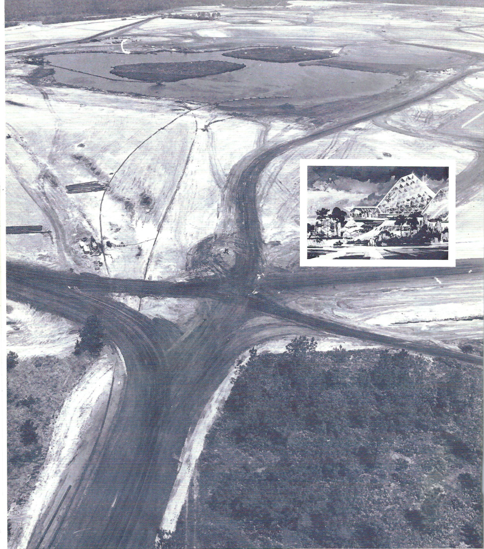
Massive job of site preparation is still going on at this tract situated between the entrance boulevard to the Magic Kingdom and Walt Disney World Village at Lake Buena Vista. A lagoon about 15 feet deep is being dredged in the center of the 200-acre site. Ground will be broken this month for the first pavilions, Energy and Transportation. Out of this barren desert will rise spectacular structures like the Imagination Pavilion (inset). (Copr. Walt Disney Productions)
